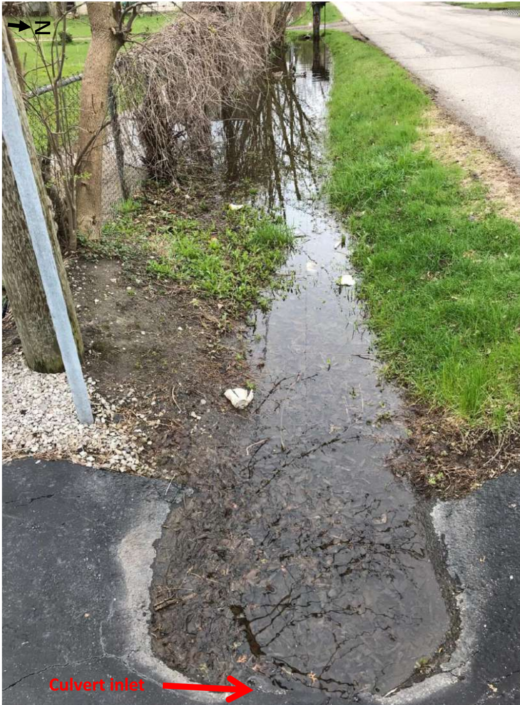
Photo taken by HRC staff on May 3, 2019 of clogged culvert inlet and stagnate water at 3185 Kenrick Street.
