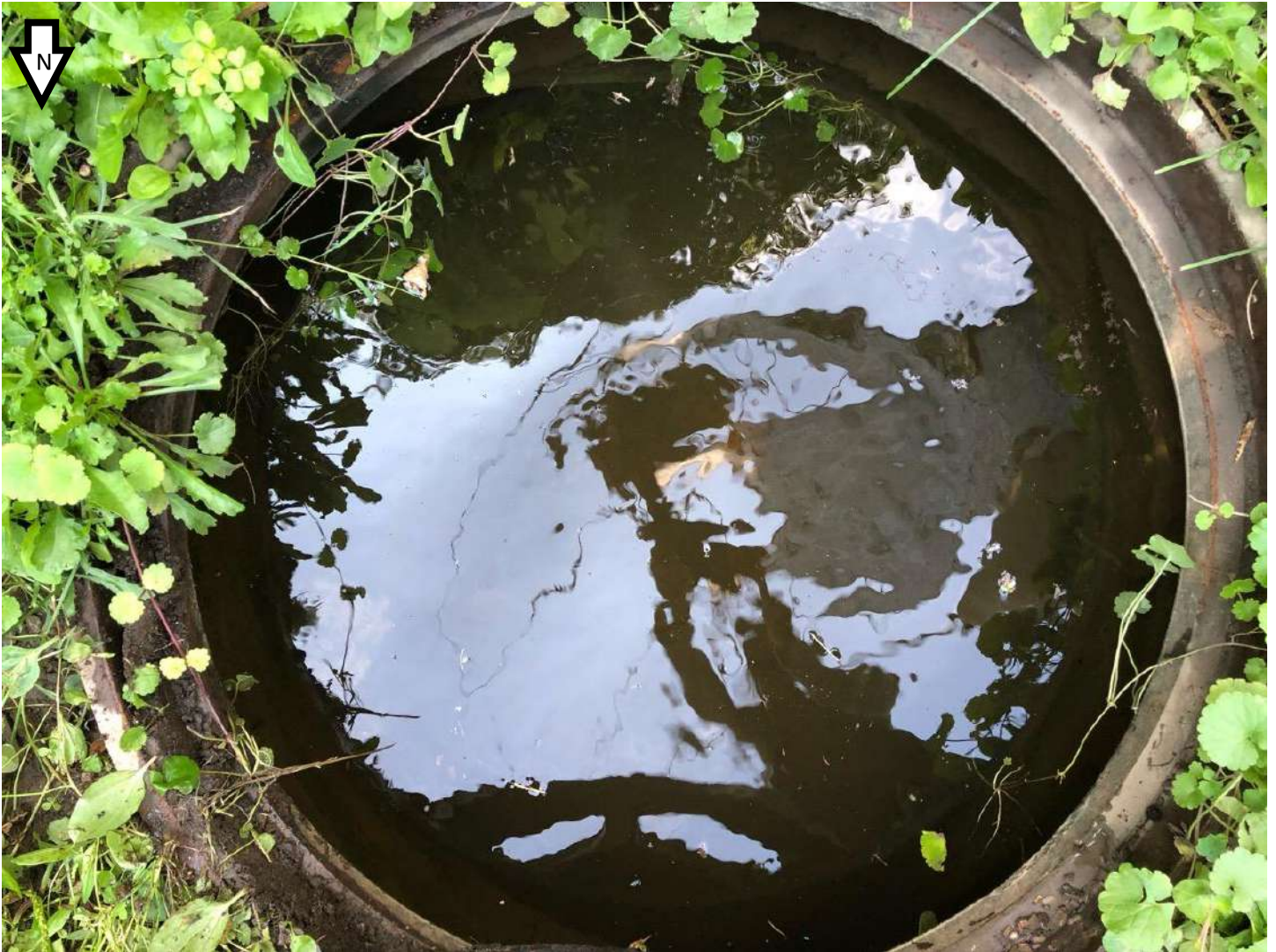
Inside image of the manhole at the end of Maddy Ln that is regularly filled with water as the outgoing pipe is below the water level in the stream.
