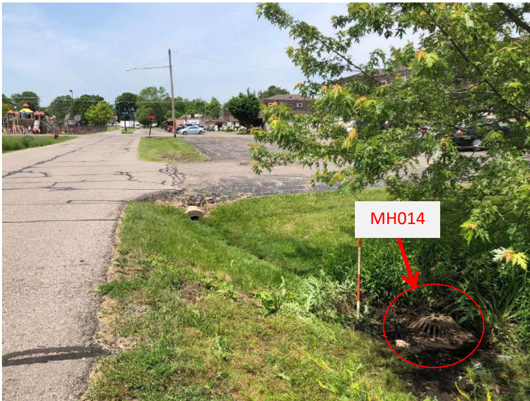
Google street view image taken in August 2018 of Schroeder Blvd., facing west and showing the location of the manhole recommended to repair.
