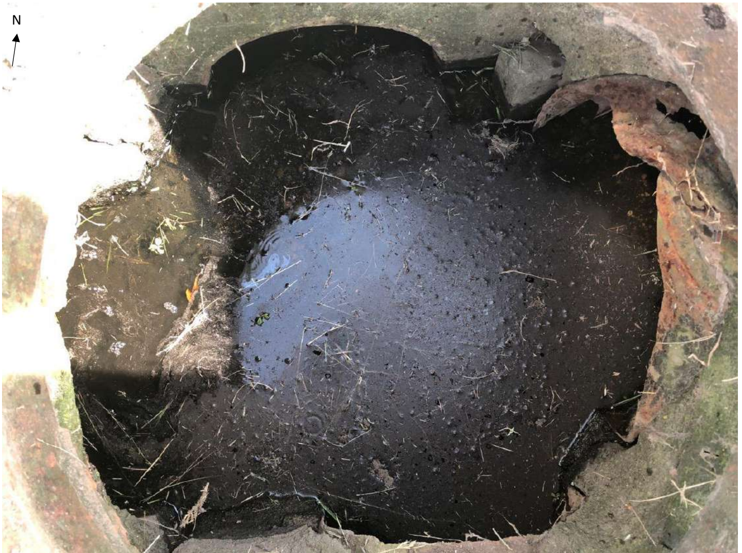
Photo taken by HRC staff on May 3, 2019 showing the inside of the manhole (MH244) at the corner of Beechmont and Schroeder.
