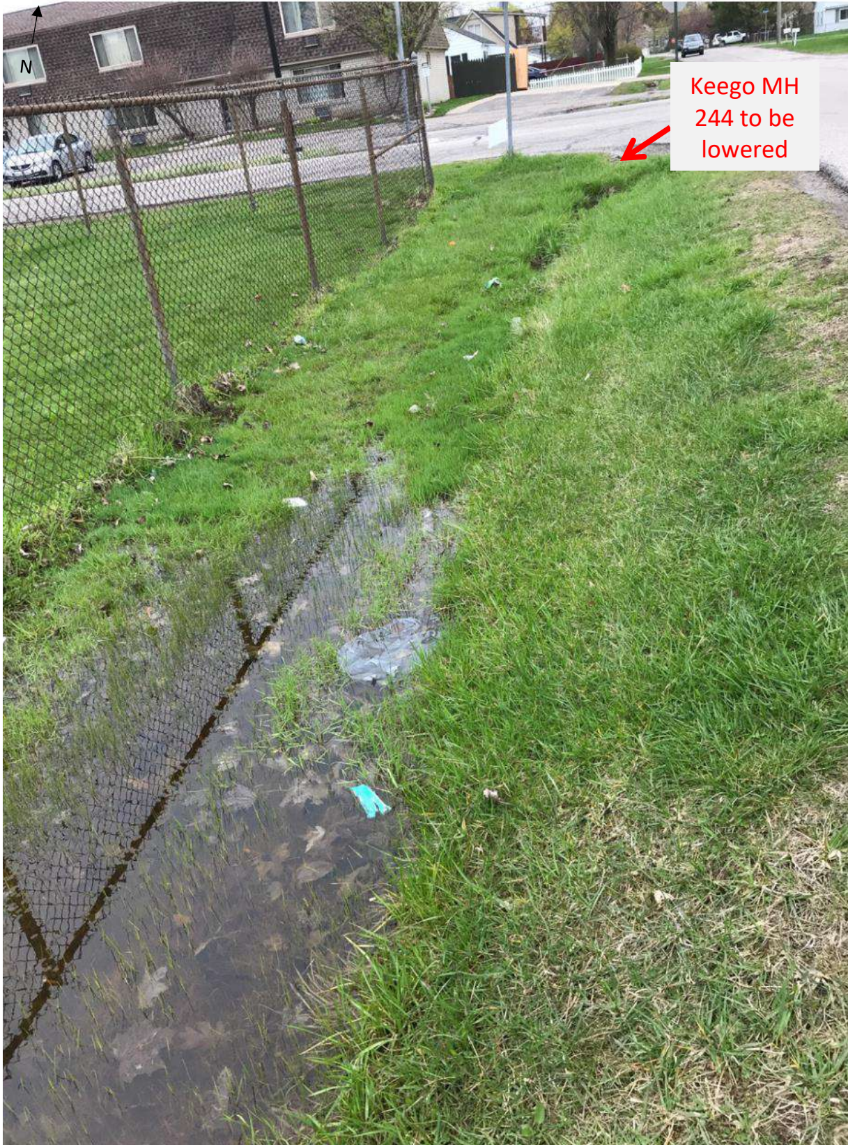
Photo taken by HRC staff on May 3, 2019 of stagnant water in the ditch along Beechmont, south of Schroeder, that's prevent flow from entering the manhole.
