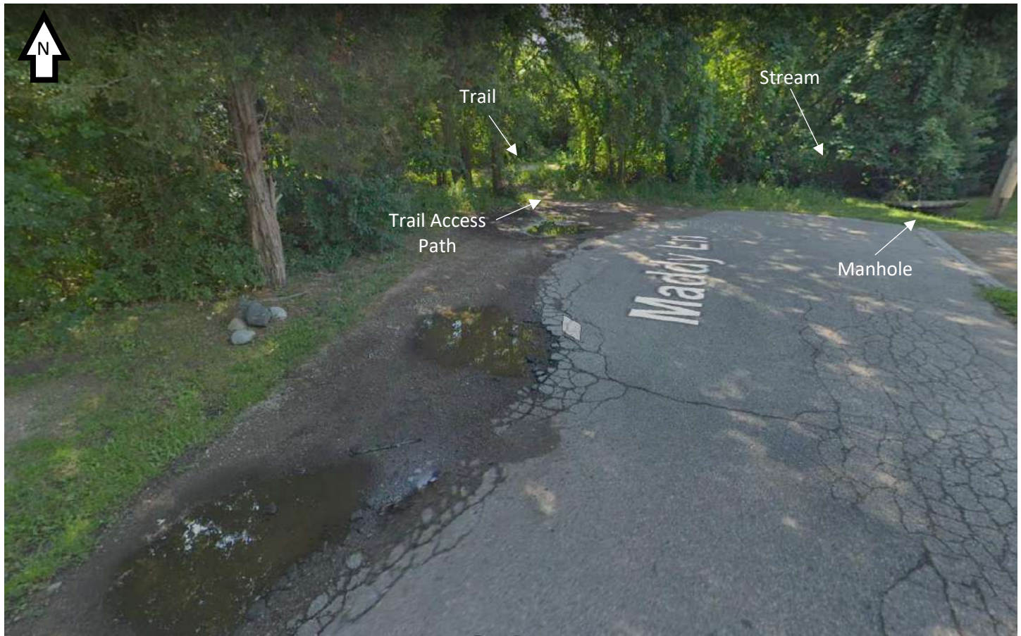
Google Street View of dead-end street where stormwater ponding occurs.
