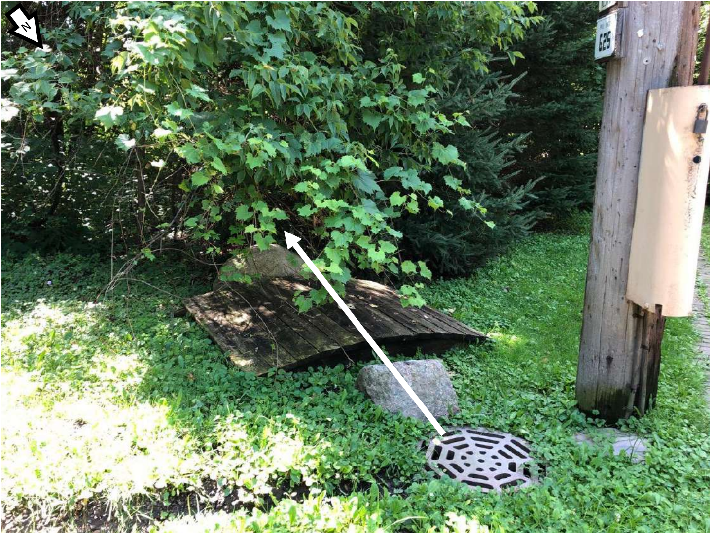
Location of the manhole at the end of Maddy Ln that discharges to the stream.
